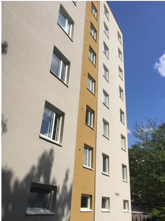
Figur 2. Fasad i ok skick.
