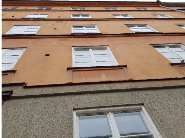
Figur 2. Fasad i ok skick.
